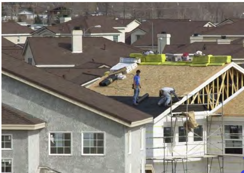
Homes are shown being constructed in NorthRidge, a Carson City residential development, in 2002. (Photo: RGJ file)
